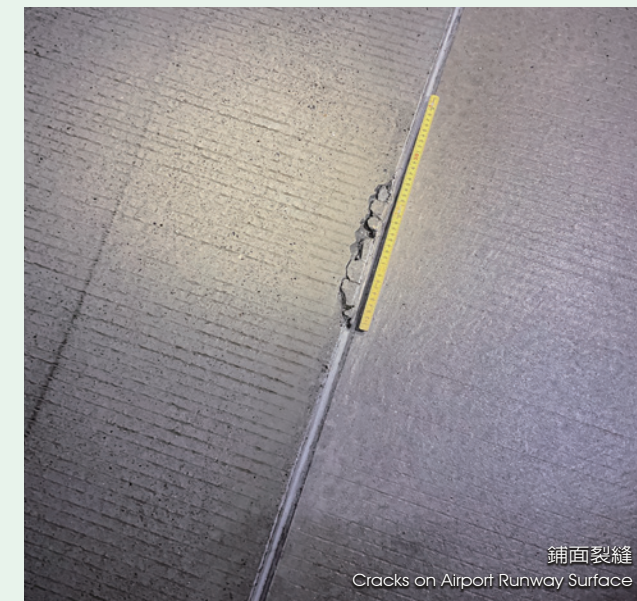
鋪面凹陷 Depressions on Airport Runway Surface
