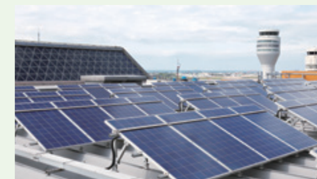
▲ 第二航廈屋頂建置之太陽能發電裝置。 Solar panels on the roof of the Terminal 2 building.
